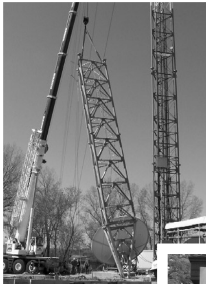
◀ WORT's new broadcasting antenna will hang about 900 feet above the ground on the new tower erected by TV Channels 15 and 57 on Madison's west side. Thanks to Ned Powell and Solidarity truckers for transporting the antenna to Madison from its manufacturer in southern Indiana.
